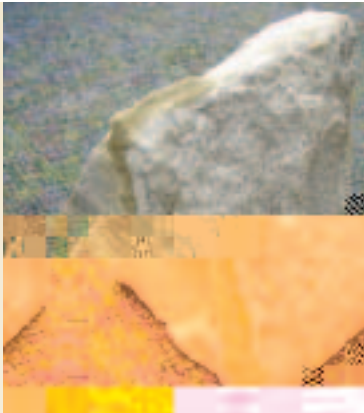
This piece of granite, removed from the chapel's north tower shows why many of the stones are working loose. "They cut away much of the back sections of the stones to make them easier to work with," project manager Don Borkowski explains. "But that left only a very narrow back section of them, the rest is gone."
